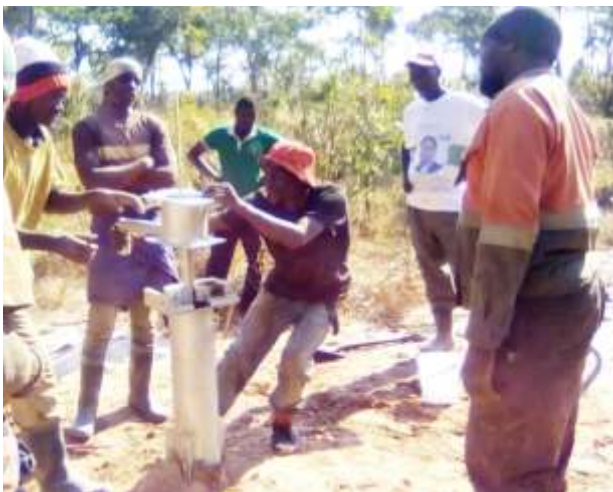
WATER IS LIFE: Workers putting up a water pump on a borehole in Mpongwe, Copperbelt Province. Providing safe drinking water, especially to rural communities, is one of our key objectives.
